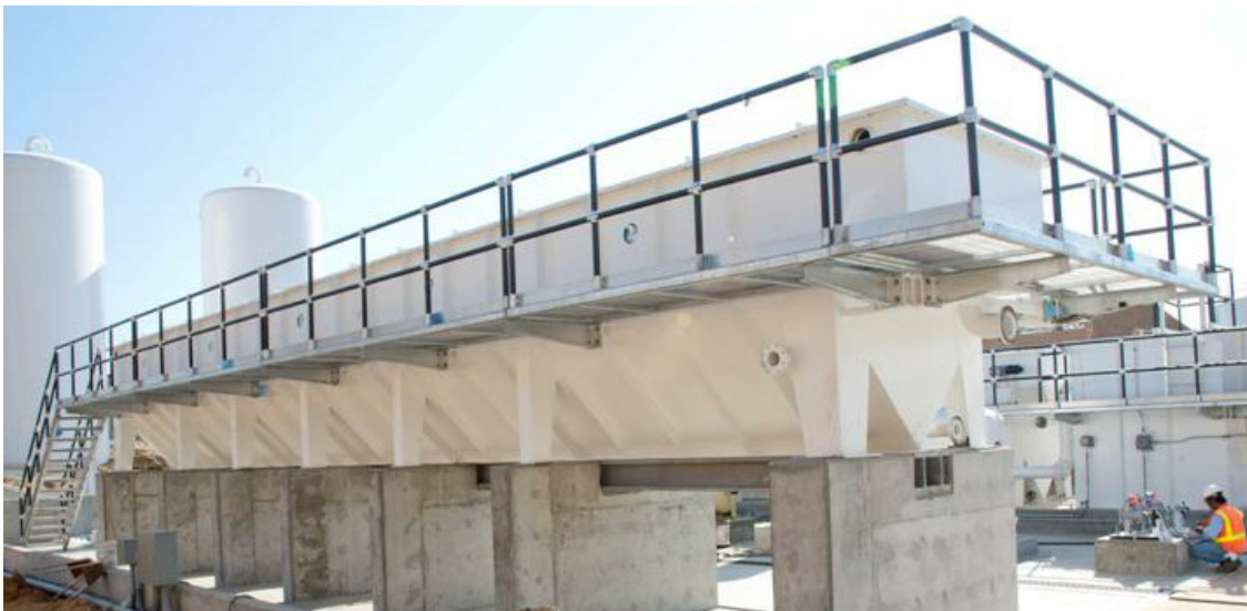
Elevated API combined with CRT chemical treatment system and DAF
