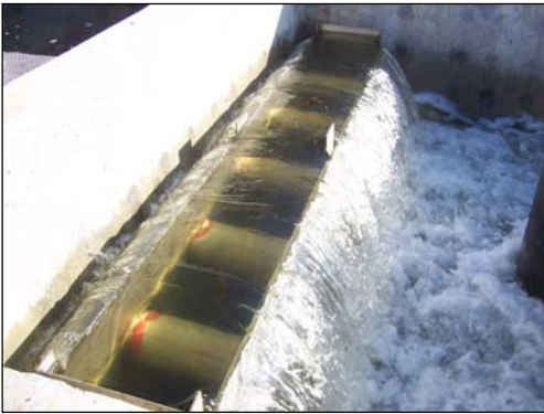
Concrete API-CPI 9,400 GPM
